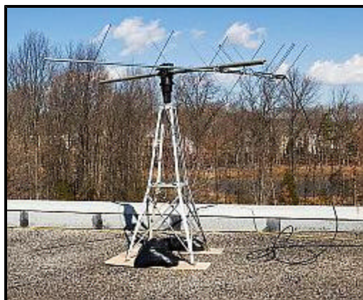
Vienna Wireless Association members installed this 2-meter antenna on the school's roof to make possible the contact between K4HTA and NA1SS. [All photographs by Linda Thomas, AC4LT]
